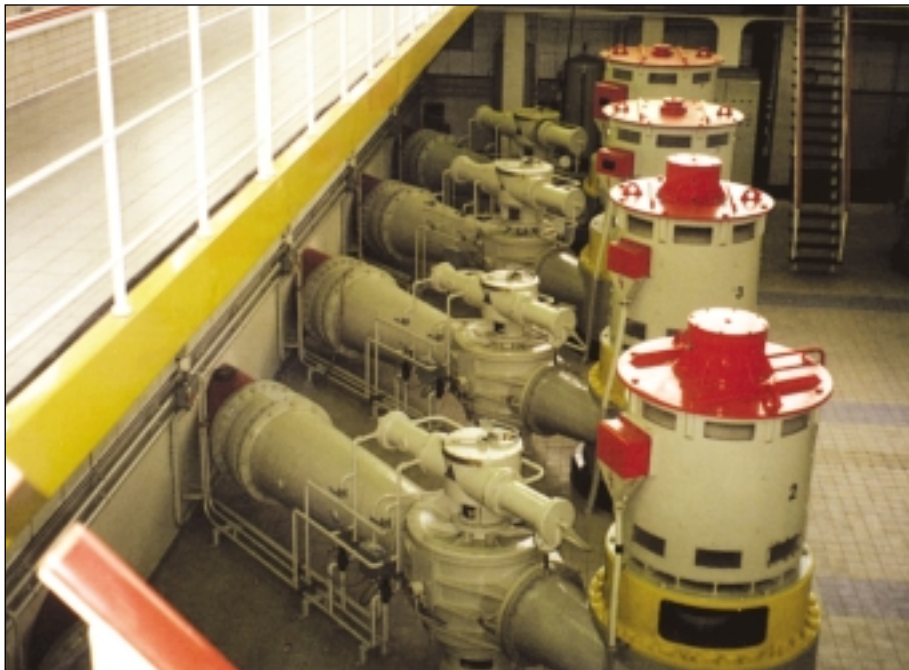
24" cone valves in operation since 1956.
