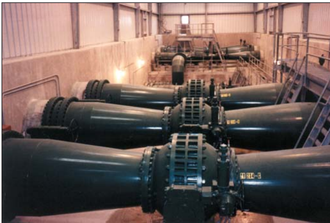
Ball valve in distribution pump station.
